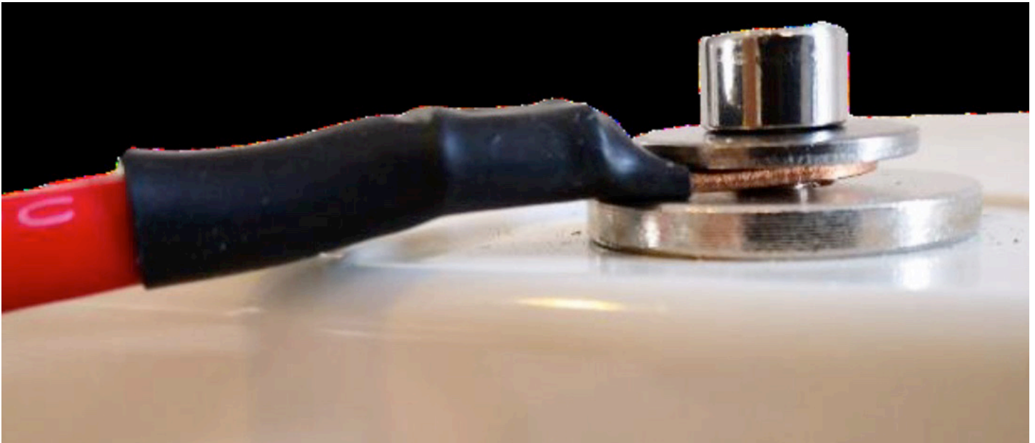
FIGURE 4. WRONG! LOOSE CONNECTION BY USING TOO LONG BOLT
