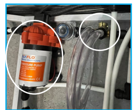
PUMP & 3-WAY VALVE FIGURE C
